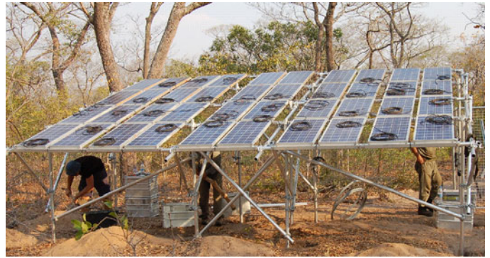
Figure 11. The 48 photovoltaic solar panels supplying energy to the equipped tower.
